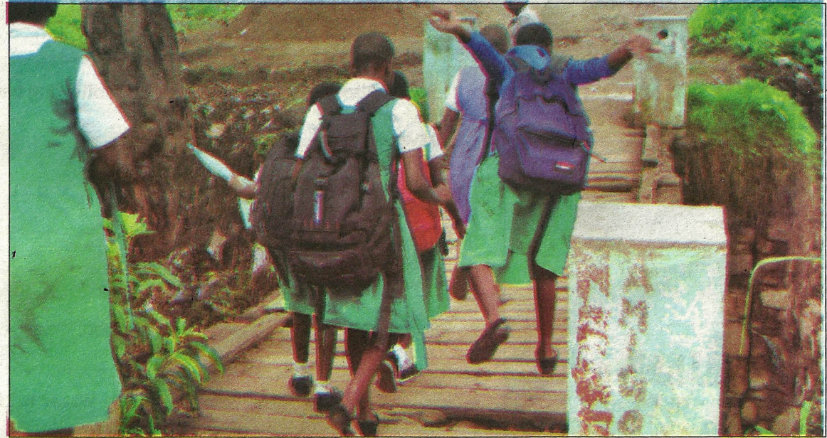
SORRY STATE—Some of Blantyre Girls pupils crossing the damaged bridge.—File picture
